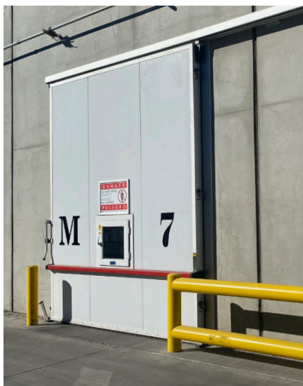
Gastight CA Door on Ext. Tilt-Up Concrete
