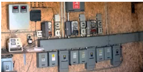
Before Kilo Watch Retrofit
